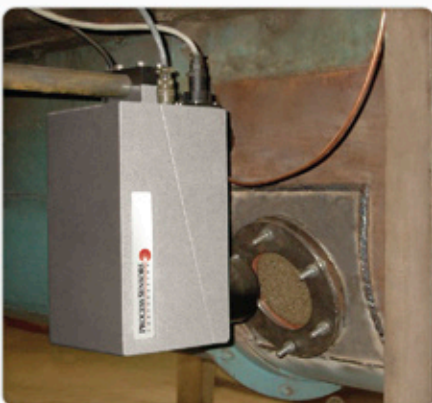
Moisture through sight glass
